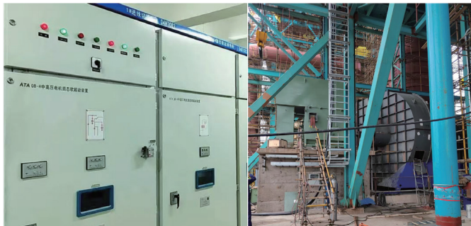
Baowu Meisteel No.4 Sintering Plant & No.5 Sintering Plant
